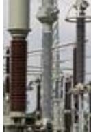
Isolators in a substation
